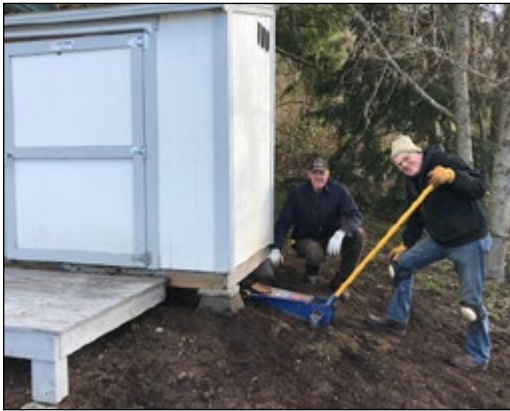
Volunteer John White, left, lead the foundation repair of the smaller book sale shed with Bill Koll's help (pictured right).
